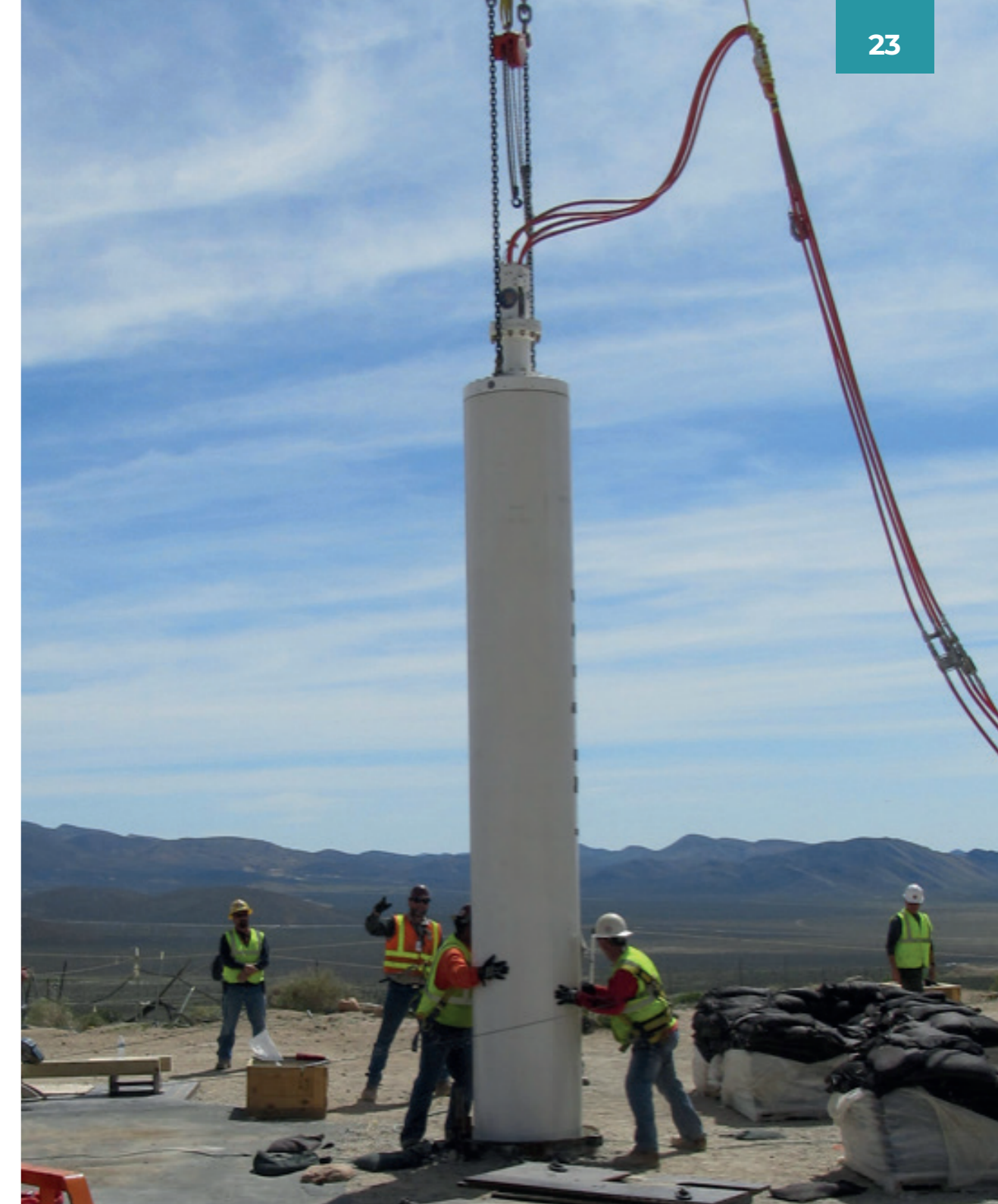
Workers at the Nevada Nuclear Security Site lower the 25-foot-long Source Physics Experiment cannister into the borehole to its center depth of 76.5 meters in preparation for a shot in 2016.
