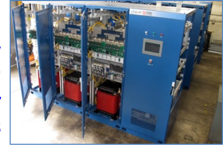
New ASIPP power supplies
