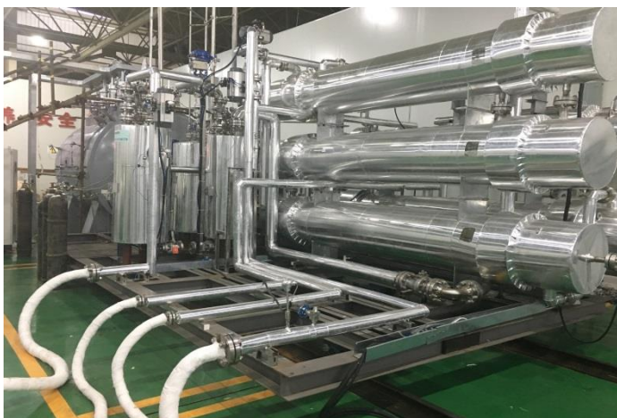
Unique HHLT facility for ITER (10 -10 Pa · m 3 /s)
